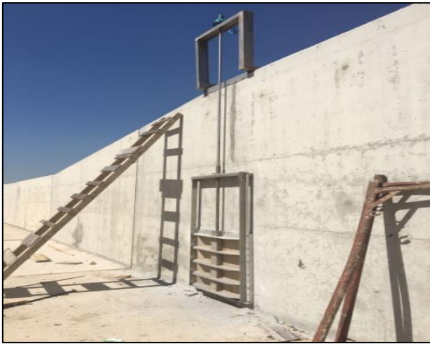
Sliding Gate at Intermediate regulator
